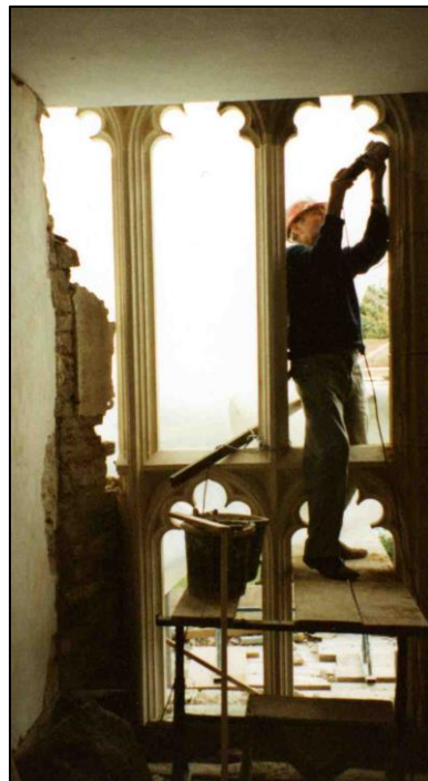
Figure 39. Restoration work being carried out on the window of the first floor bedroom in the west end of the former nave, (south elevation of church)
