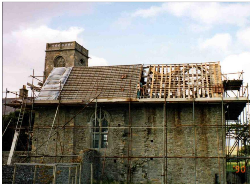
Figure 31. Further repair was required to the infirmary roof in September 1990.
