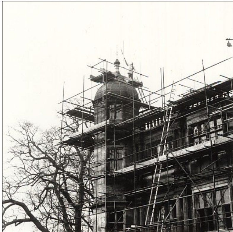
Trying out the stem of the new weathervanes on a repaired cupola.
