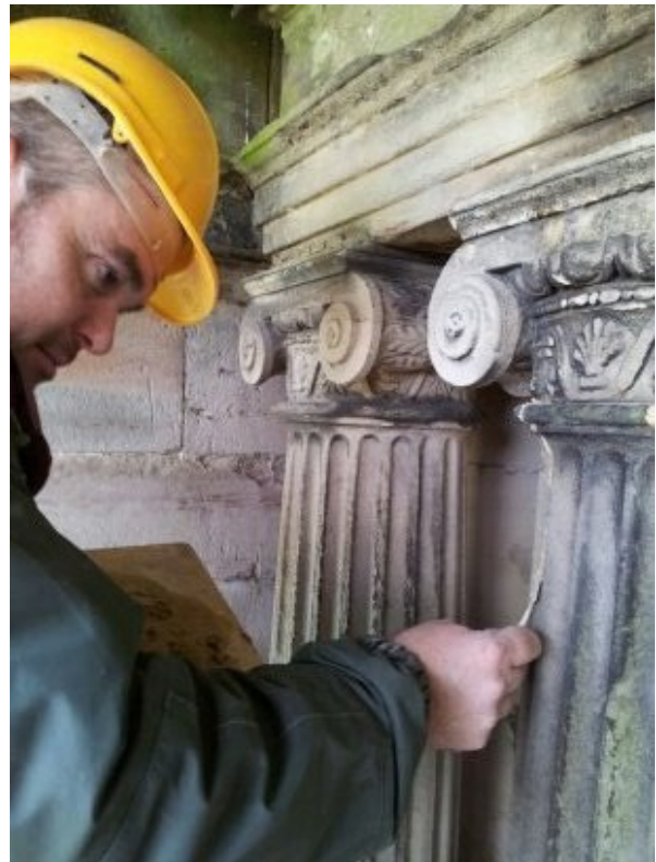
Cracking in the carved stonework called for fine grain filling with lime mortar.
