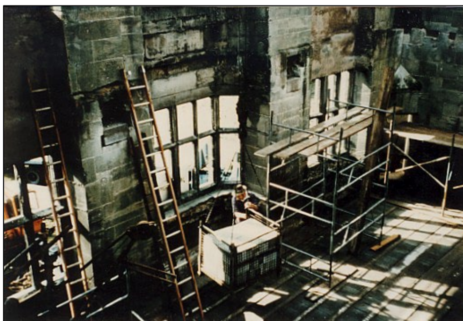
The first floor is complete, but materials for now can still be lowered by crane through the open roof and upper floor.
