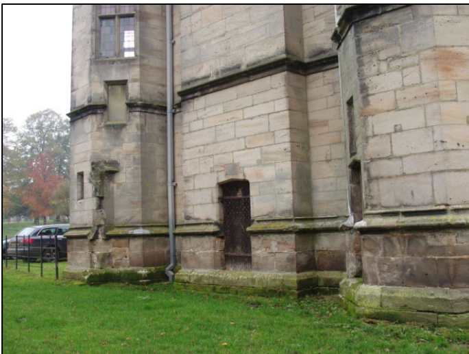
Examples of anomalies at Tixall: top blocked doorways on ground and first floors on the east elevation, with masonry scars where earlier walls were keyed into the Gatehouse; bottom,
