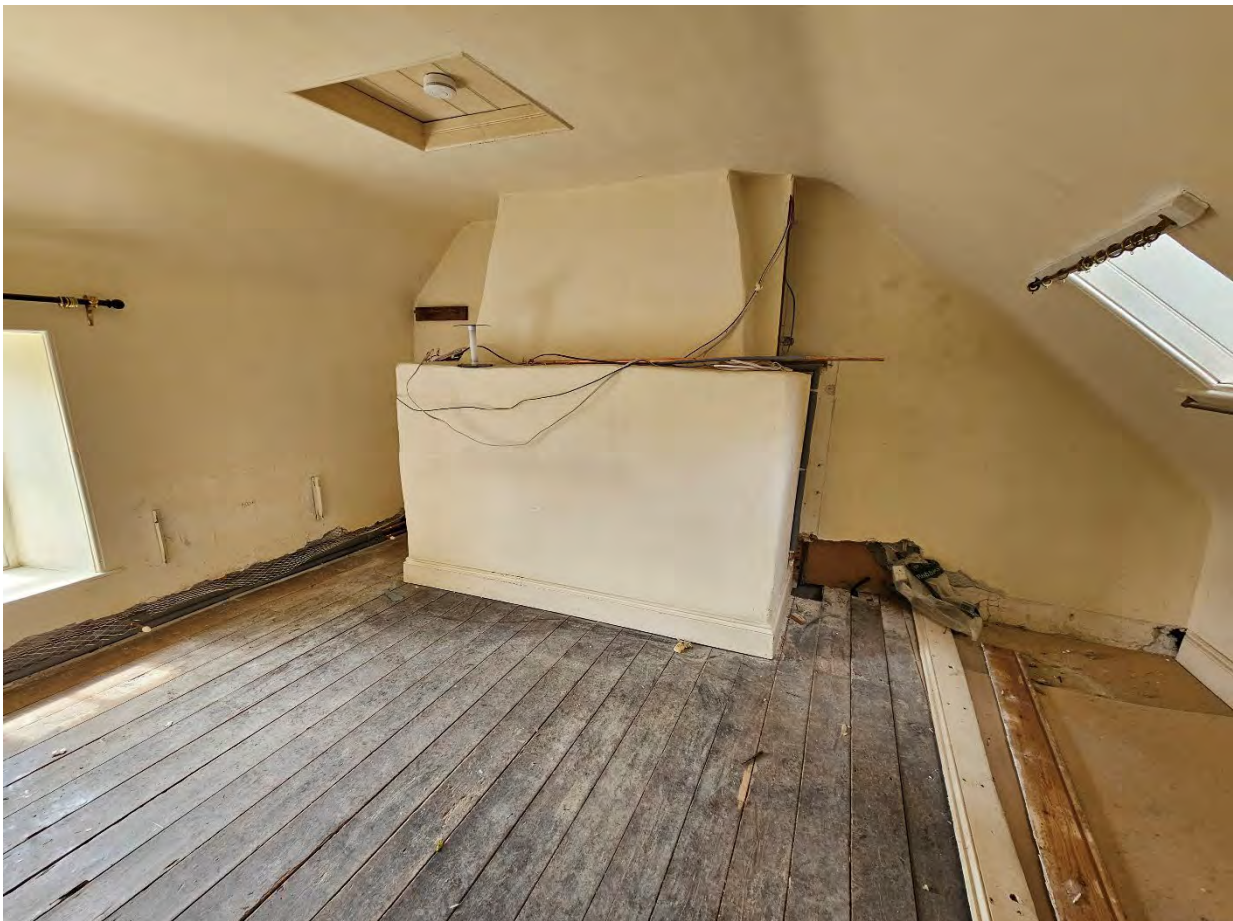
The first-floor chimney breast on the problematic west gable in the Farmhouse. The porous granite of the walls was allowing water penetration; the roof space above was poorly ventilated.
