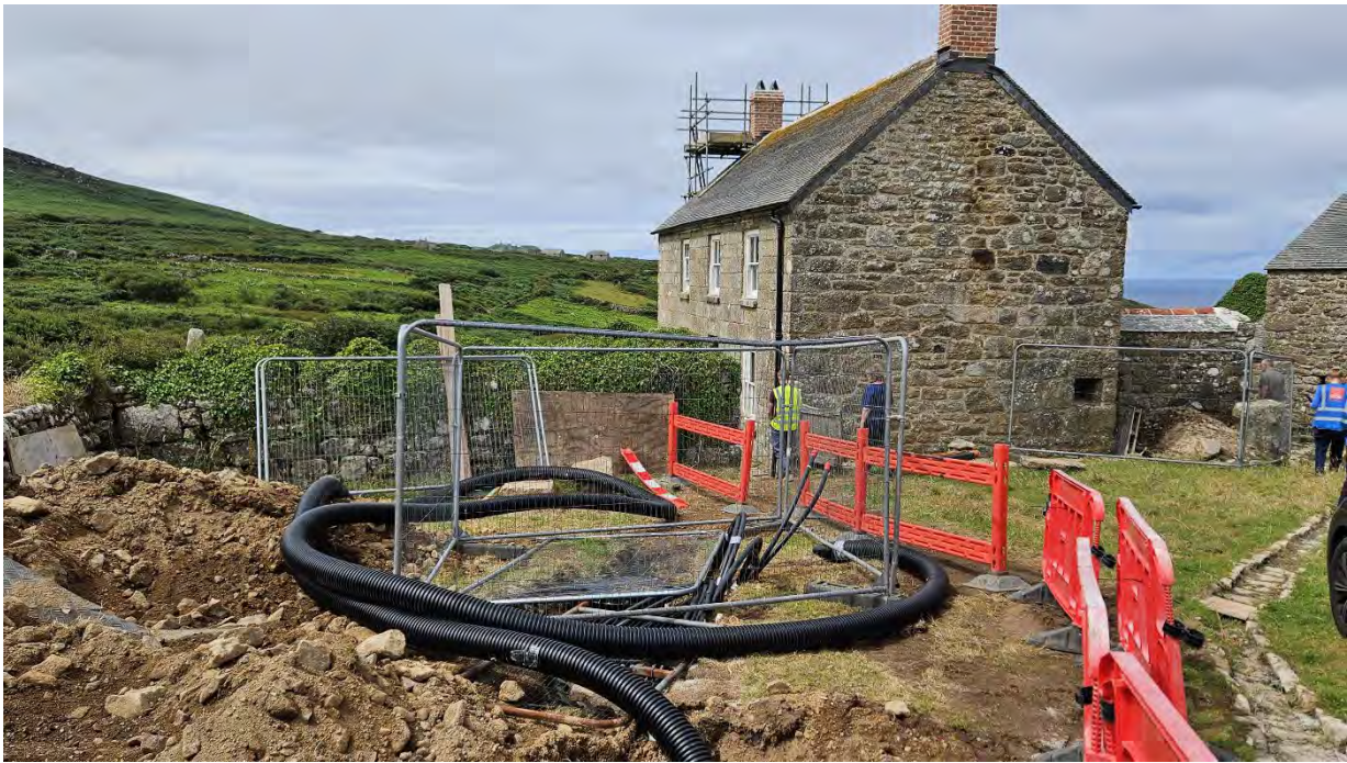
The Farmhouse during the 2024-5 works, with just some of the ducting and groundworks required for the new ground source heating installation.
