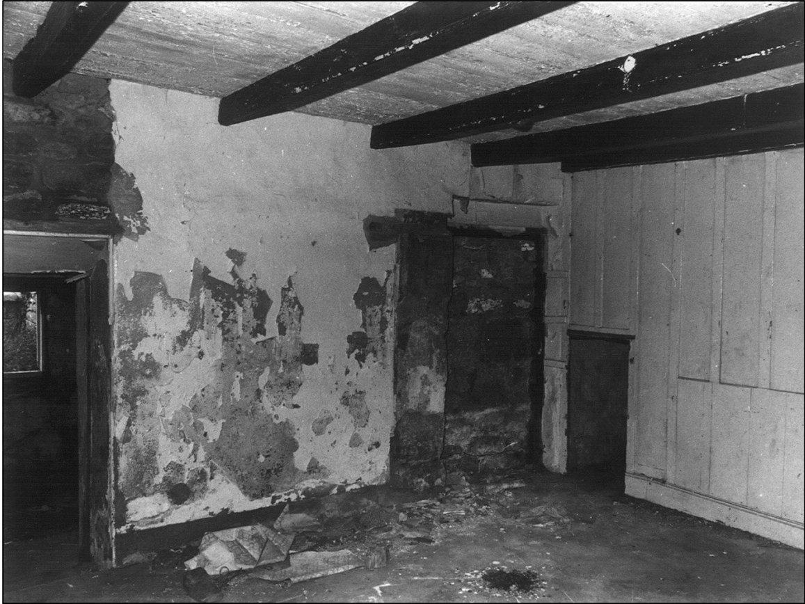
The Farmhouse: the door into the yard had been blocked but its frame was still intact. All that was needed was a new door. The wooden partition dates from the building of the house c. 1800. The floor once made up of old mill-stones, on top of which concrete had been laid.
