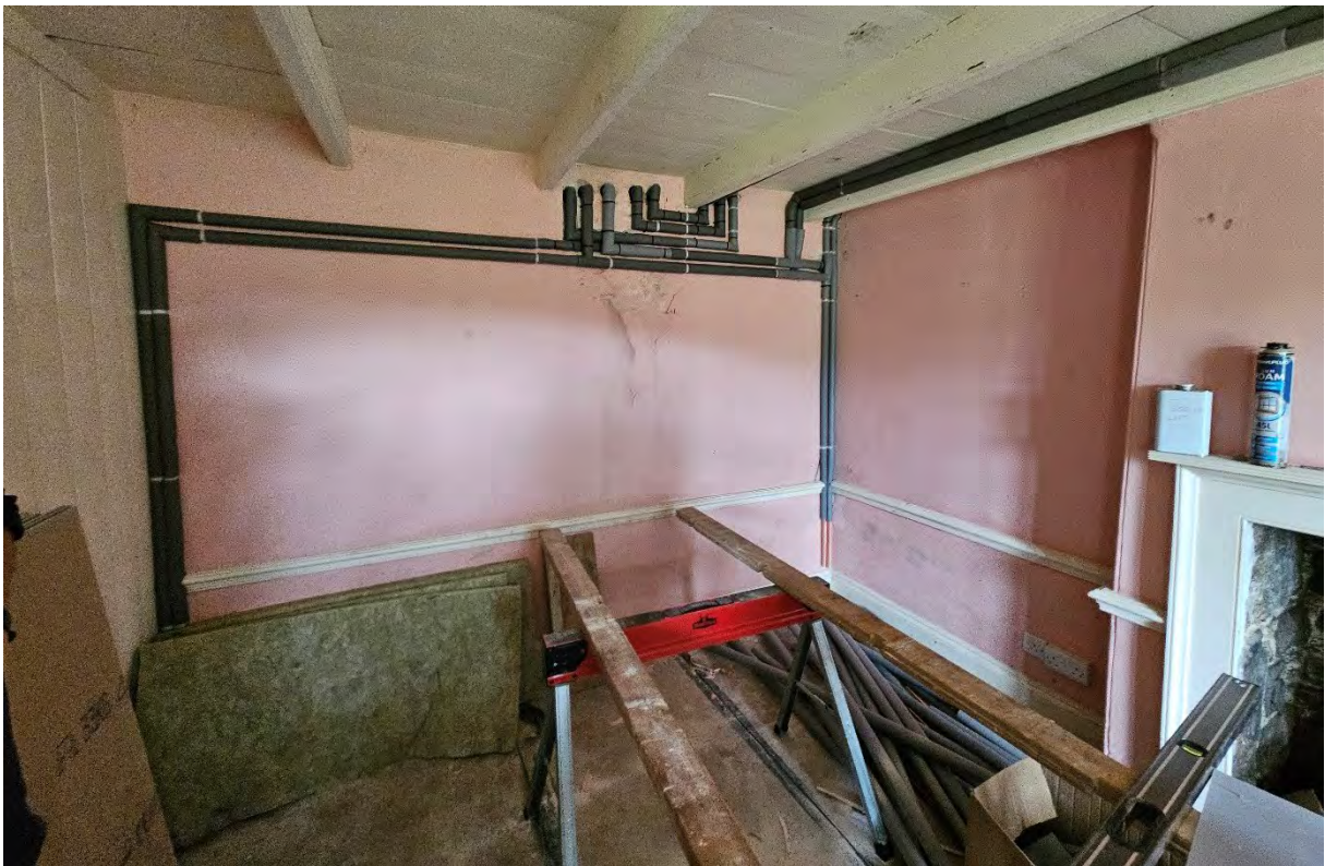
Work underway to transform Captain's former kitchen into a sitting room, including sound deadening to the joists; and the new pipework in the sitting room at The Farmhouse.
