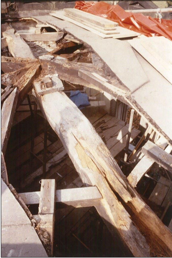
Main roof beam exposed
