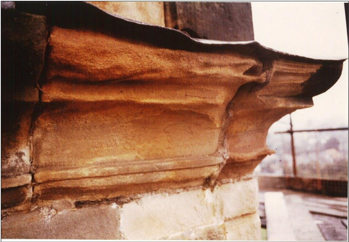
Condition of main cornice stonework, before
