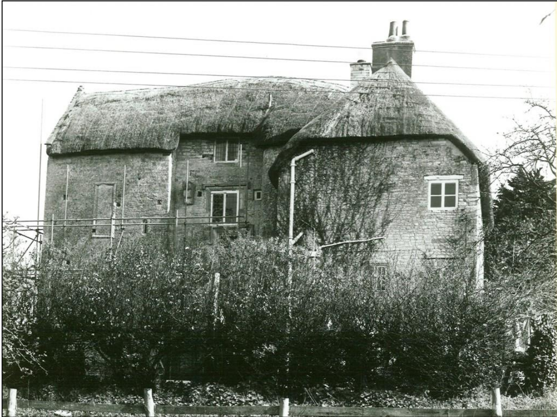
The north end in 1978. The late 18 th century window beneath the 17 th century drip mould can be seen resting on the head of the restored medieval window, thus weakening the wall. The retaining arch over the window has now been fully reinstated.
