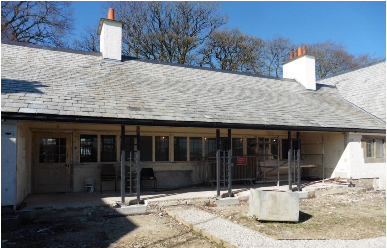
Top: the new canopy framing in place and awaiting glazing. Below: re-landscaping, with the veranda trellis supports reinstated.
