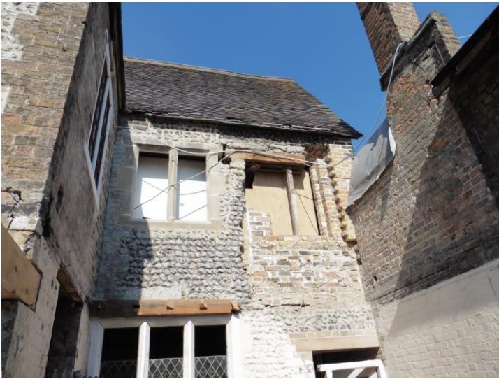
The south elevation takes shape. Top: view of the reconstructed service range roofs from the scaffolding; middle: the south elevation stripped back ready for repair; bottom: the oriel window newly in.
