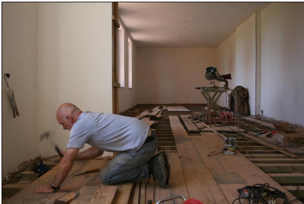
Laying the floorboards salvaged from the London docks, autumn 2007. By now, the whole room has been plastered out.
