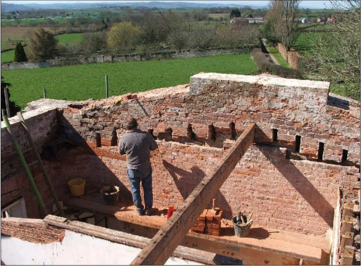
Repairs underway to stabilise the west pediment. This was right at the beginning of the restoration project in 2005, when new roof timbers had yet to be installed to replace the rotten ones, already removed here.
