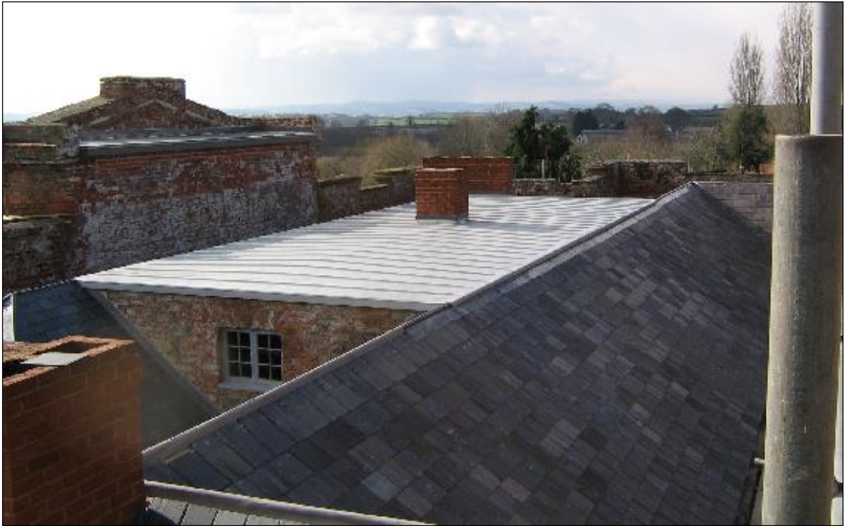
View southwest across the south range in March 2005. The roof of the south range is curious in design. A valley roof might be expected of its double pile; instead, the roof running back from the portico is almost flat.
