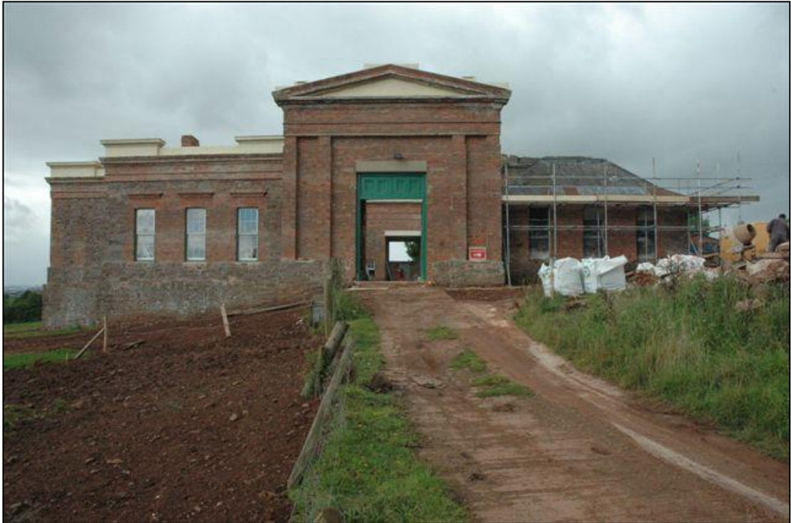
The east range in August 2007, with scaffolding up to rebuild the northern parapets.
