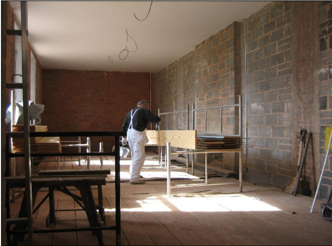
March 2007: painting the massive skirting boards in the south range. The large openings for carriages between the brick pillars have been blocked up in and a new flue inserted in unmistakably modern materials, and are waiting to be plastered.
