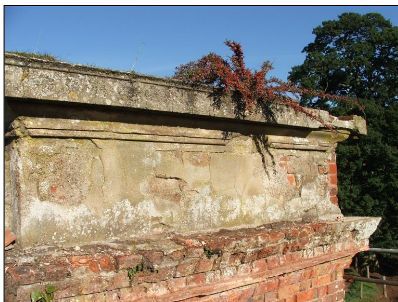
Surviving render at cornice level on the parapet on the south elevation – the famous patented metallic cement.
