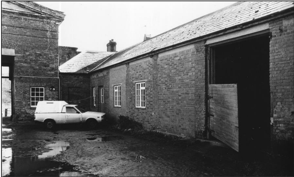
Courtyard side of the south range before work began, showing how the doorways into the carriage houses had been bricked up.
