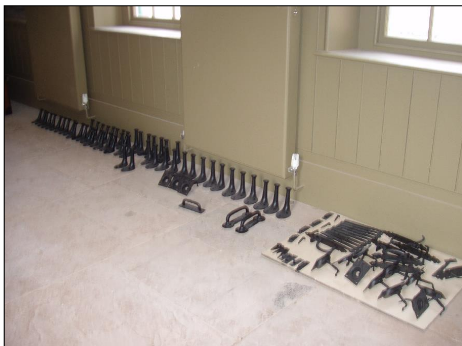
Cast iron tack pegs and door furniture reproduced from originals, waiting to be fitted beneath the fully opened tack room windows in March 2008.
