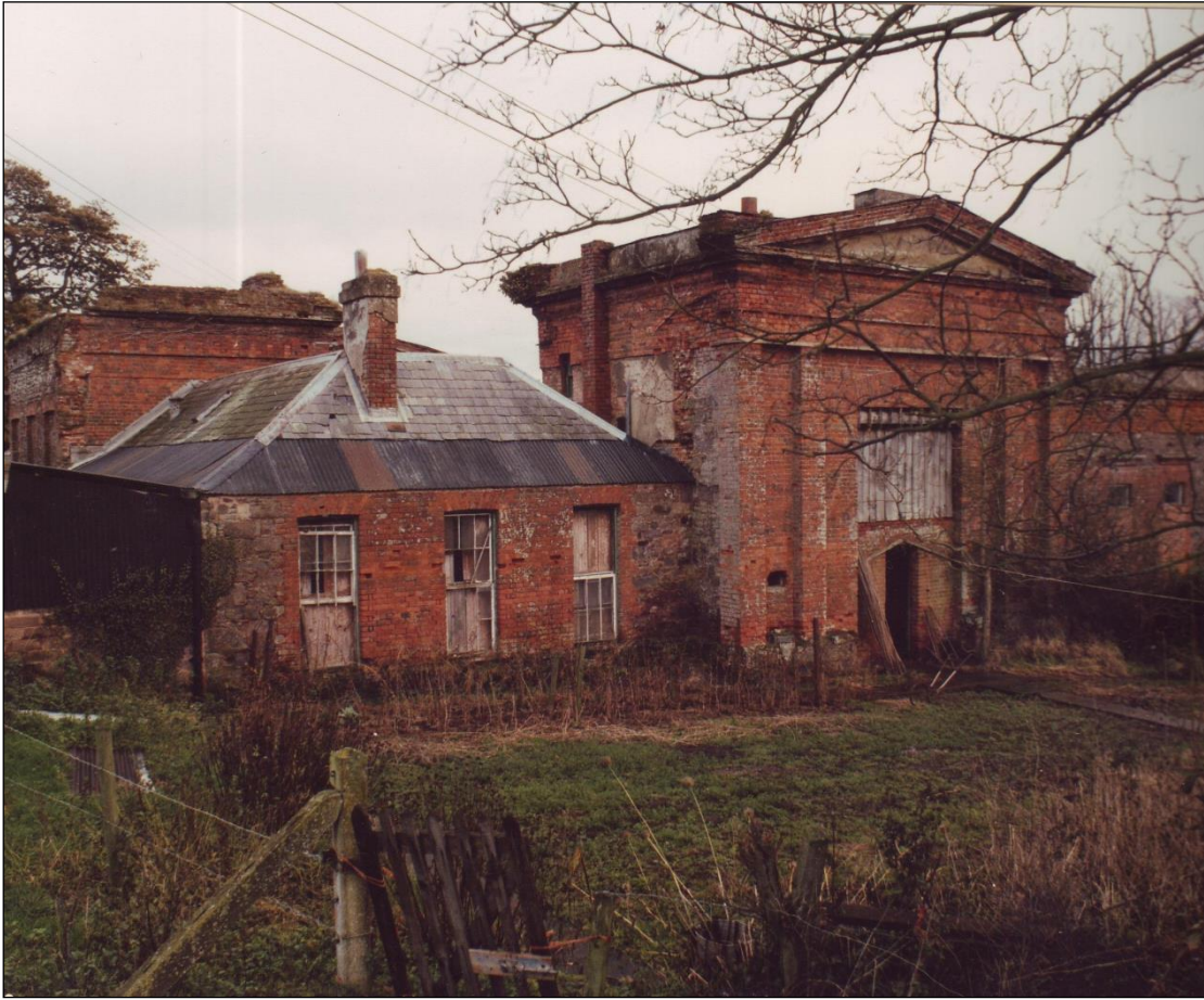
The west range before work began. The parapets on this northwest corner have been lost, and the roof patched in with corrugated iron.
