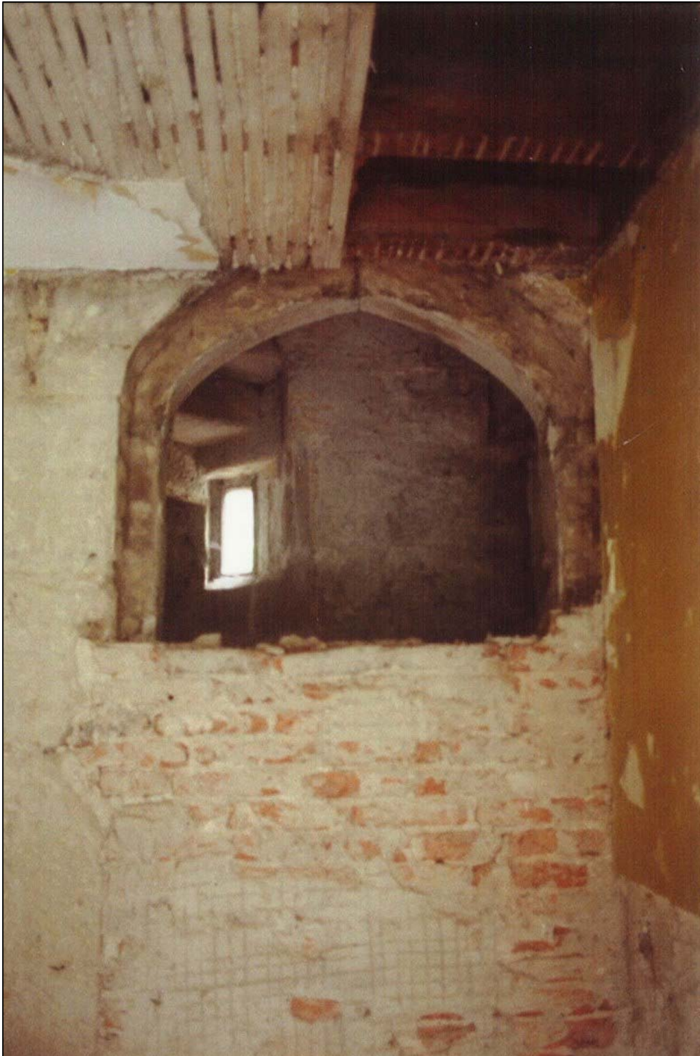
Opening the original doorway from the spiral stairs to the second floor, December 1990.
