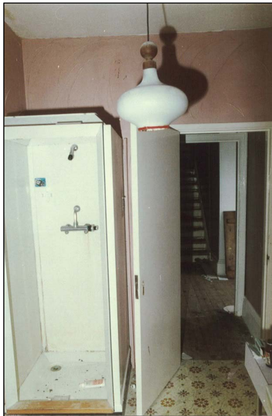
Shows cabinet in present bathroom and old stair (19 th C) up to attic.
