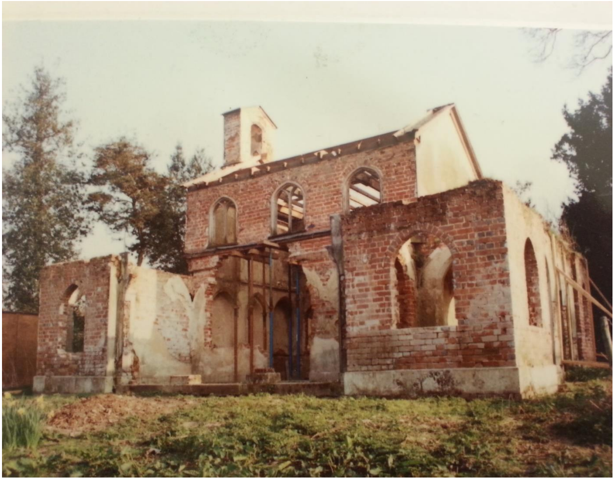
Cobham Dairy in 1983, stripped back ready for re-roofing and repair of its shell.
