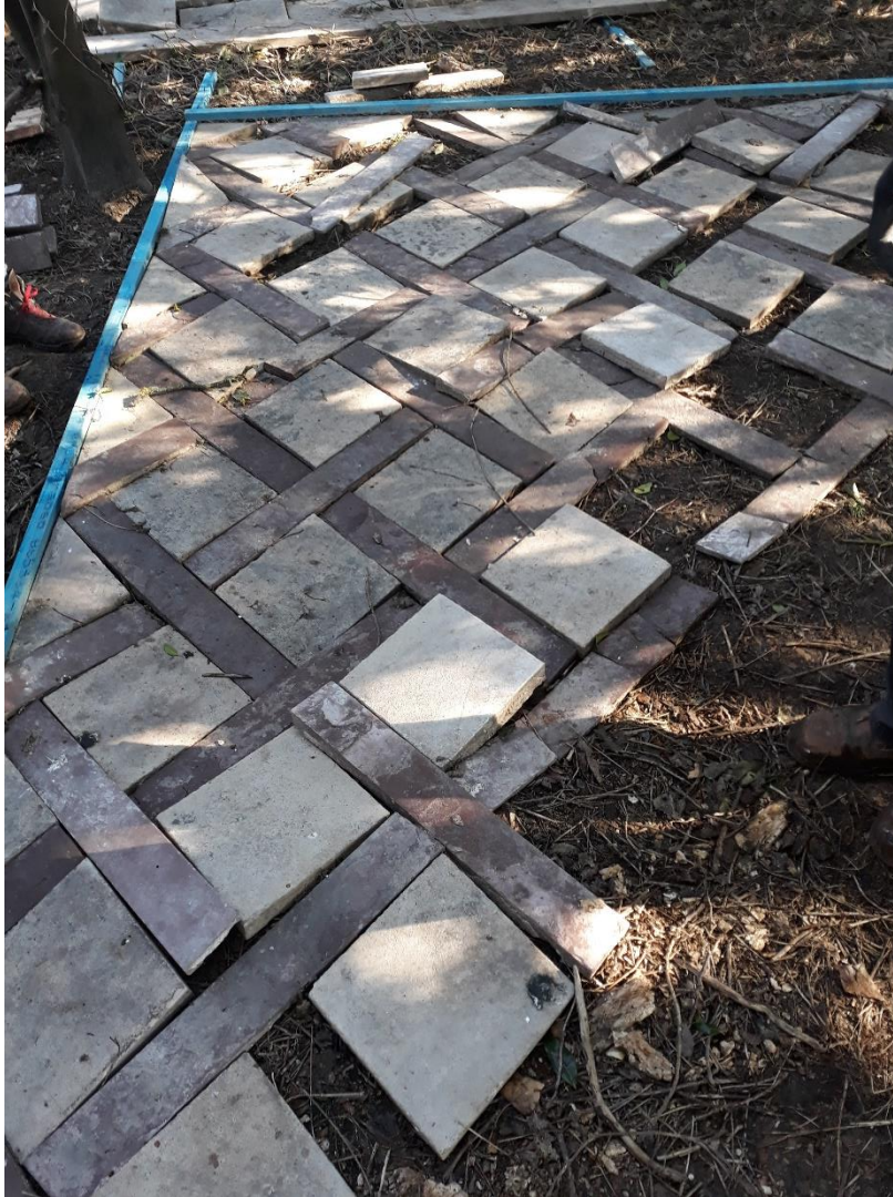
Laying out the salvaged floor in the main chamber, removed to install the underfloor heating. It's unclear whether this was laid in the late 18 th - or 19 th -century; either way, it is another fine feature of the building.
