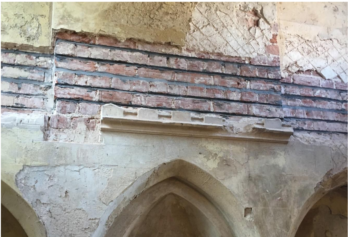
The north and south clerestory walls were found to be bulging and had to be taken down and rebuilt. Metal ties have been concealed between the brick courses for added strength.
