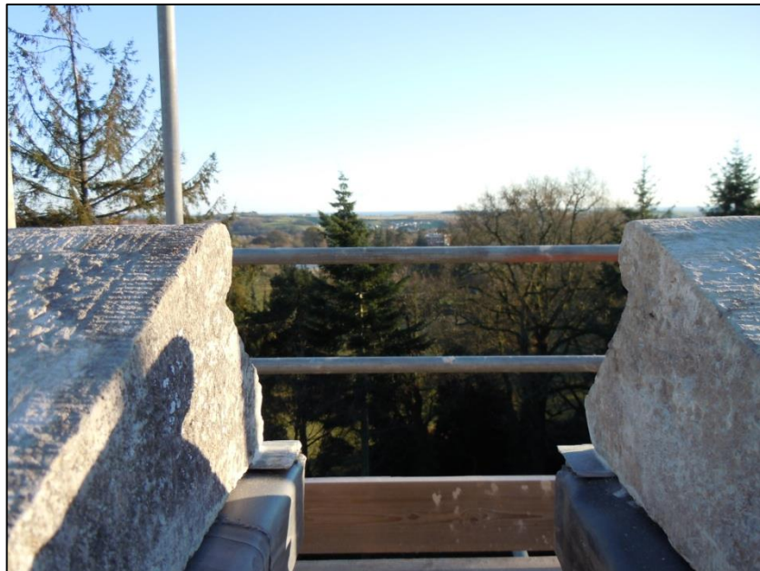
The careful tooling on the blocks of Ashburton marble that form the high level roof copings suggest they were intended to be left exposed.
