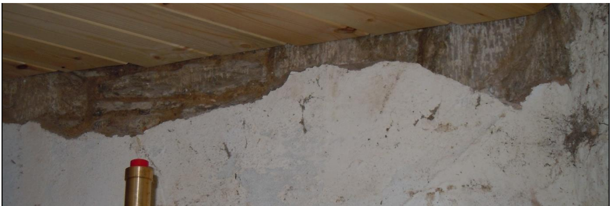
Fair face stone revealed behind plaster in the service block, that led site manager Brian Berry to speculate that the whole tower might once have been exposed stone.
