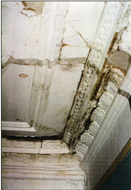
The plasterwork on the landing ceiling was in a bad state
