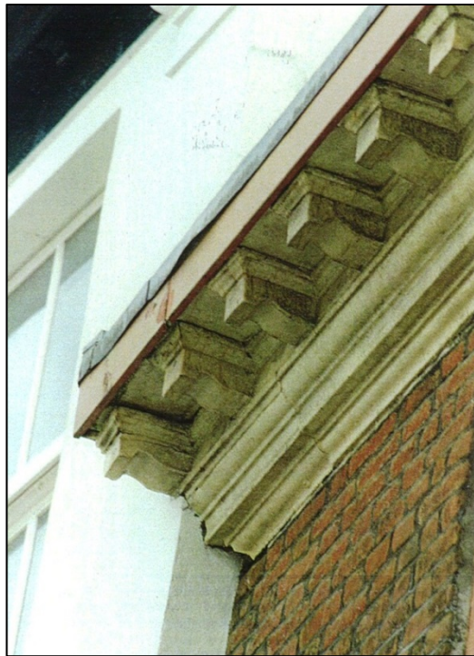
The top mouldings of the cornice had been replaced by a red board
