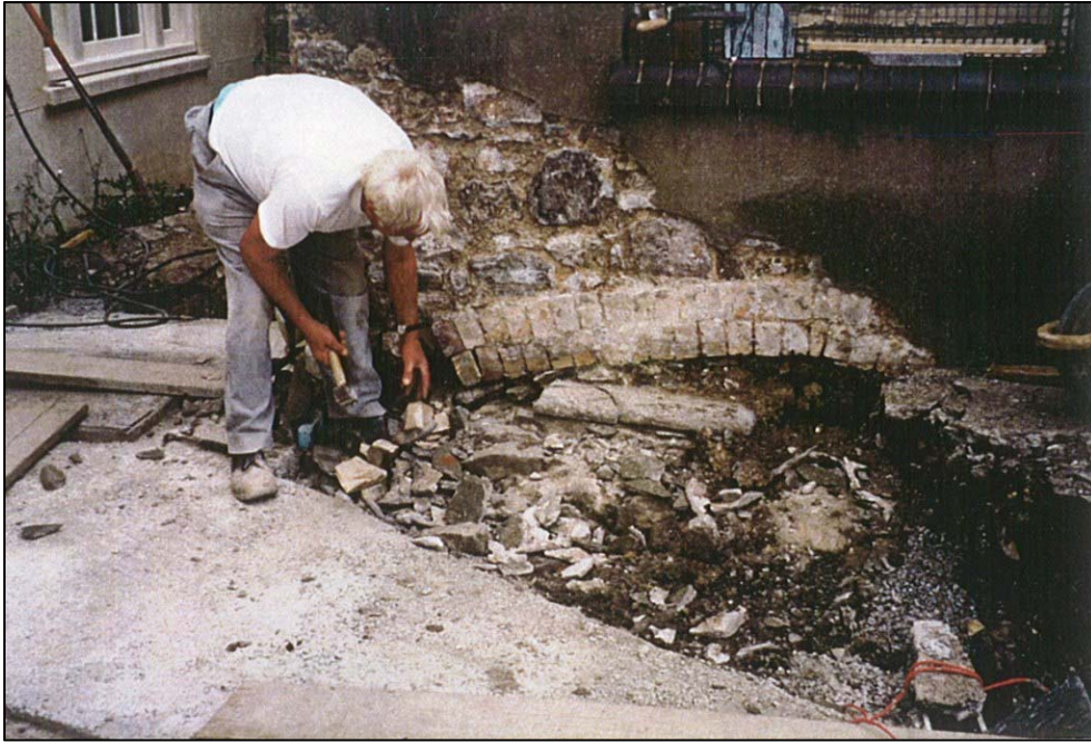
The well being discovered beneath an arch under the cloakroom when it was demolished
