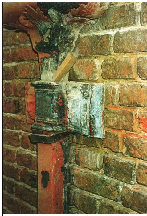
The downpipe at the front of the house needed repair
