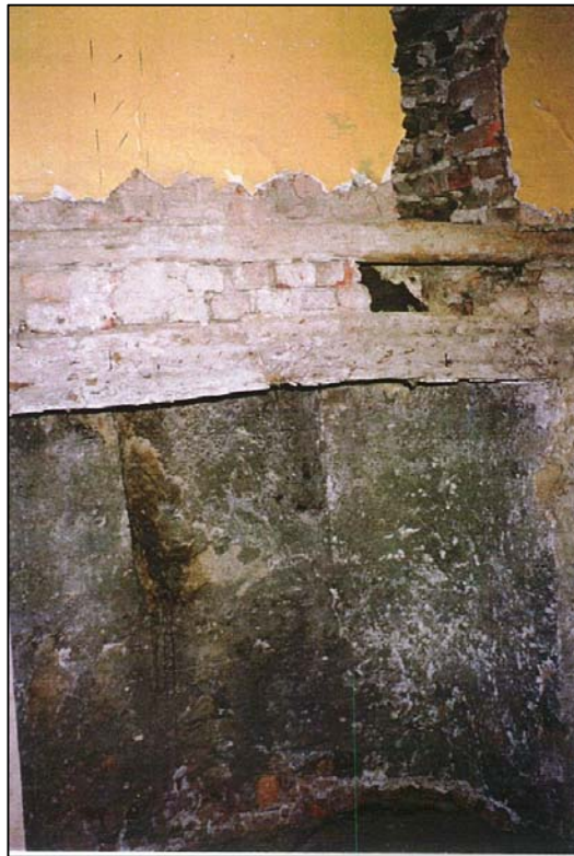
A kitchen fireplace was found in the present kitchen on the north wall
