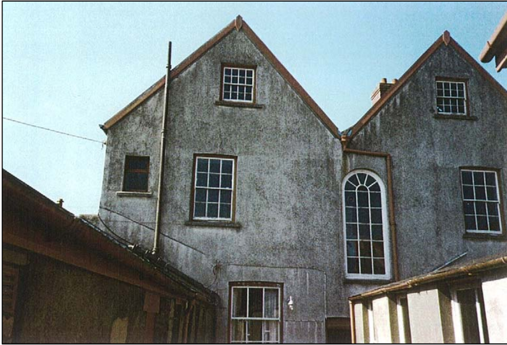
The back of the house as found – the downpipes have been replaced and the sheds removed
