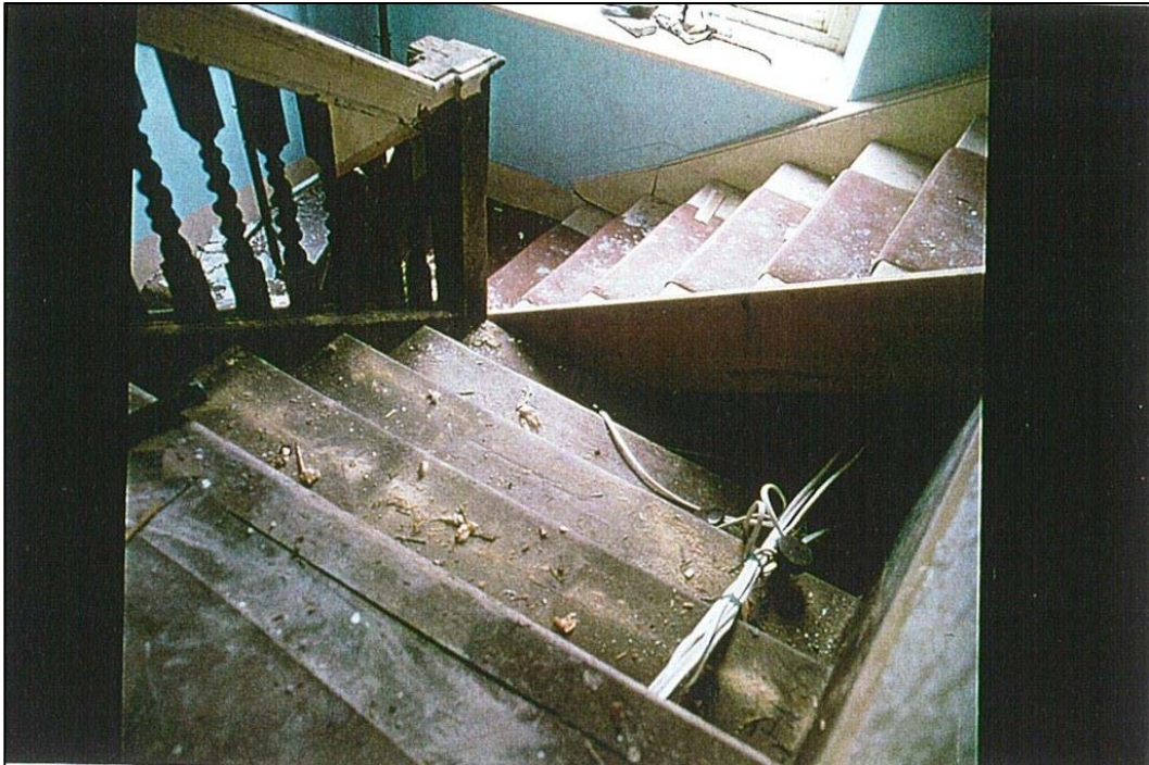
The main staircase with the additional flight put in by the Freemasons
