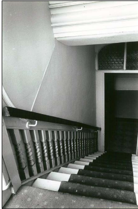
The first flight of the main stairs. The stair well is boarded up on the left and the original handrail can be seen behind the new one.
