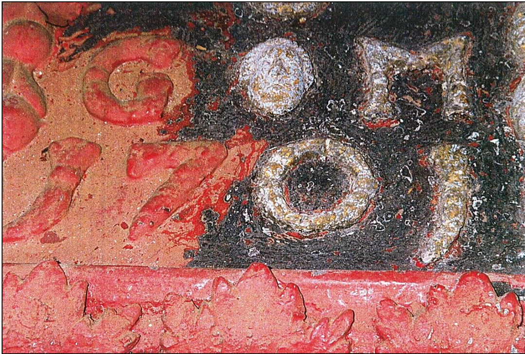
A drainwater hopper: beneath the red paint there was gilding, then the original grey to which it has returned
