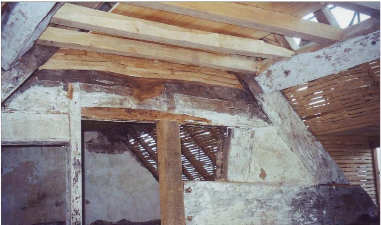
Honest repair: a new doorpost tenoned to the first floor truss. Hand riven lathes were used to reinstate the wattle and daub ceiling. The ceiling timbers were green oak cut from the neighbouring wood. All internal timbers were originally limewashed.
