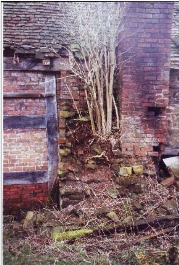
The bread oven, shown here externally, had collapsed.
