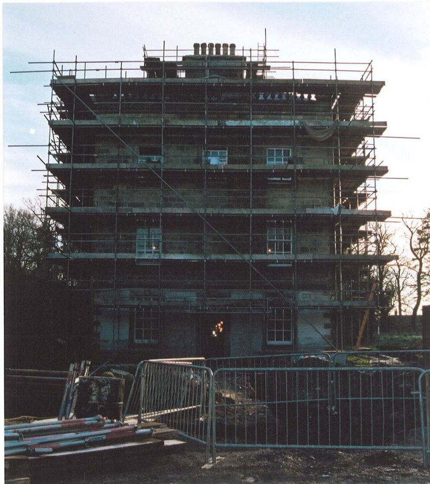
The east and north elevations of Auchinleck House, February 2001. The scaffolding was up throughout 2000 and the first half of 2001.
