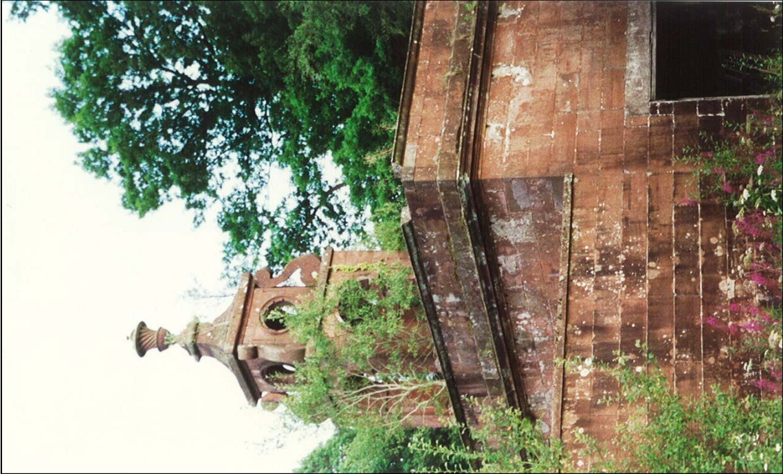
The north west pavilion before repair
