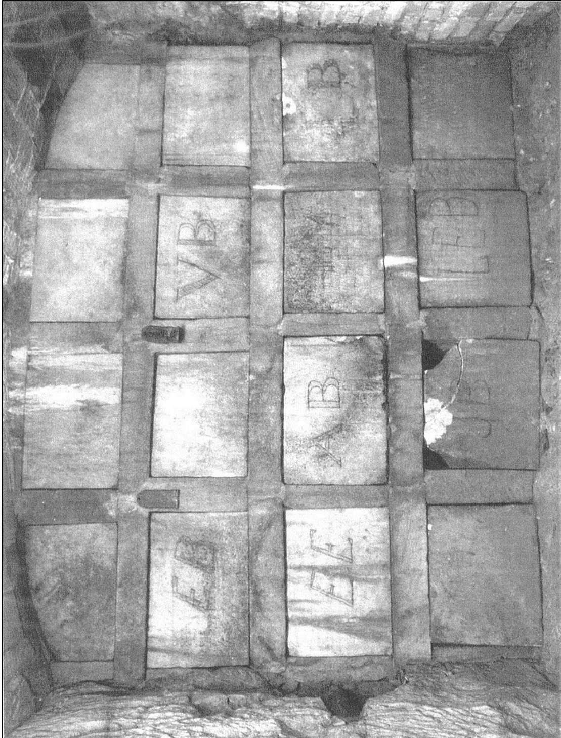
The Boswell family mausoleum in Auchinleck. The vault is easily accessible and holds a series of stone shelves identified with the initials of the deceased
