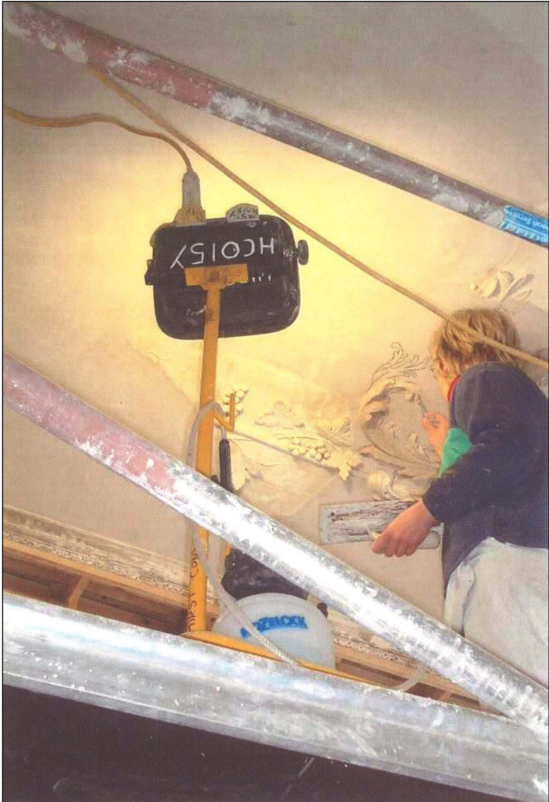
A specialist from Clivedon Conservation working on the plasterwork on the dining room ceiling.
