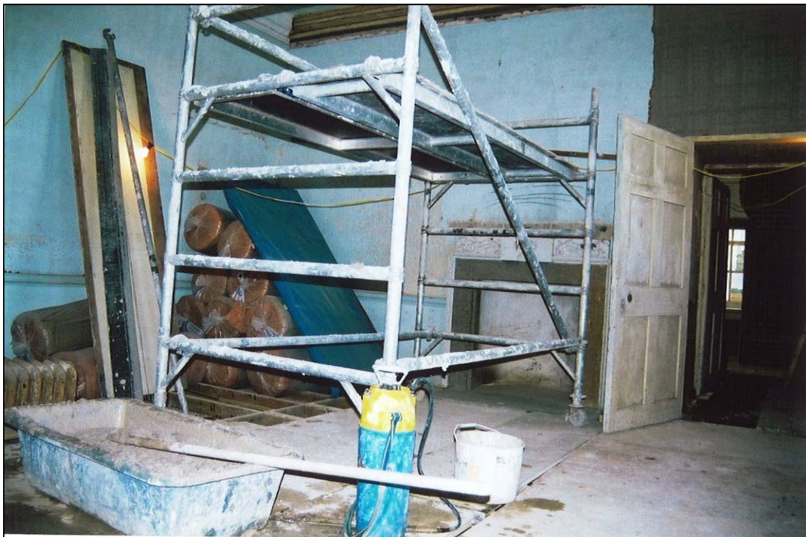
The principal bedroom on the ground floor, February 2001. The floor has yet to be relaid; a trough of lime plaster is curing in the middle of the floor. Much of the original plaster has been saved. A new scratch coat is drying over the door.
