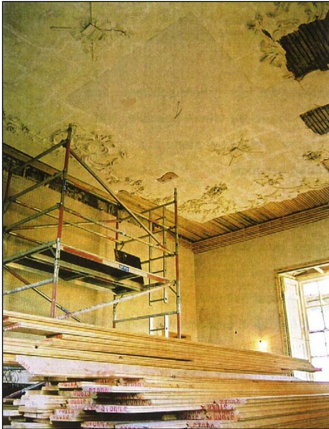
The dining room in February 2001. The ceiling perimeter had failed through water damage and the cornice is almost missing. New flooring planks are waiting to be laid.
