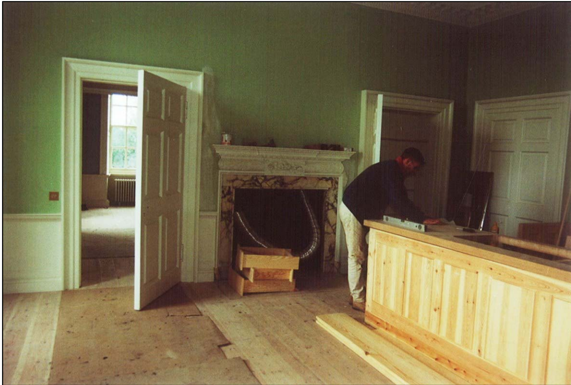
The kitchen nearing completion, the newly discovered wall cupboard and blind door to the right.
