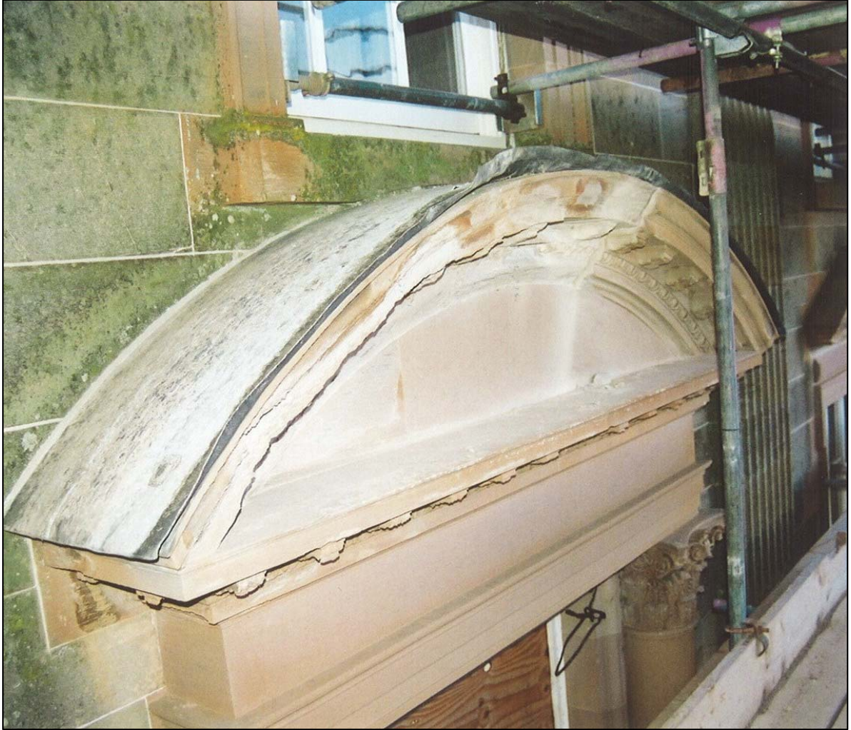
The moulding over the lintel of the front door was badly eroded by the weather.
