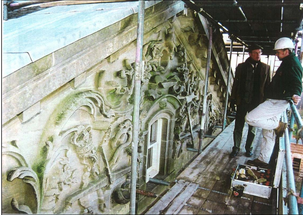
Architect James Simpson and stone conservator Nick Boyce discuss the consolidation of the pediment.
