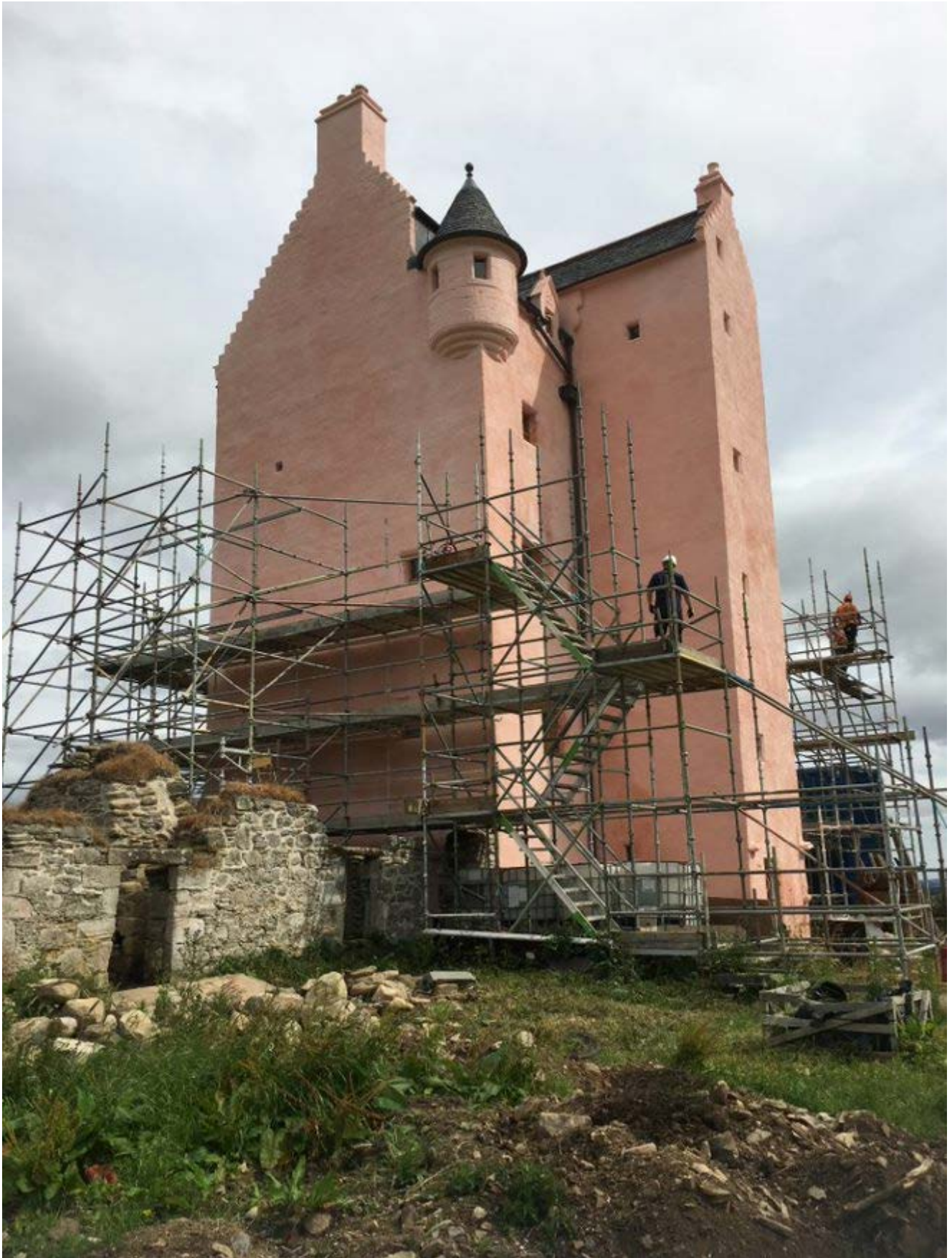
By August 2022, the tower was finally emerging from its chrysalis of scaffolding.
