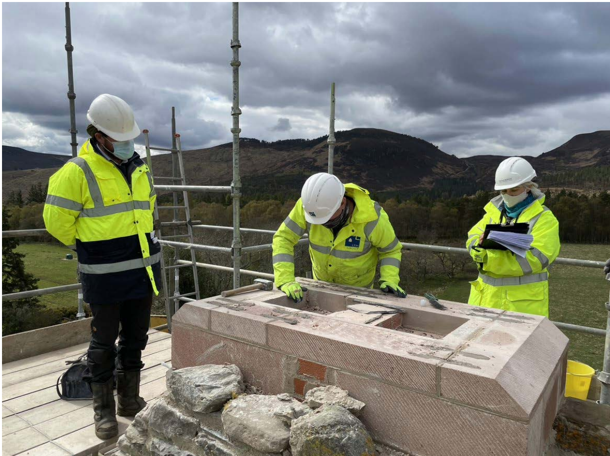
By summer 2021, masonry repairs were well underway onsite (top). Inspecting a new chimney flue carefully built around the surviving stump (below).
