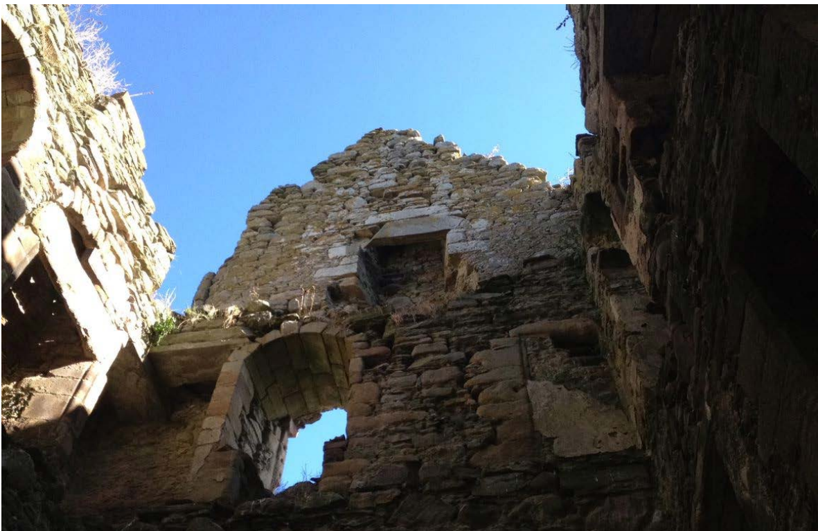
Inside the gutted, floorless shaft the tower stood open to the sky, its walls tantalising covered with features waiting to be interpreted. Remarkably, there was still plaster clinging to the walls in some places.
