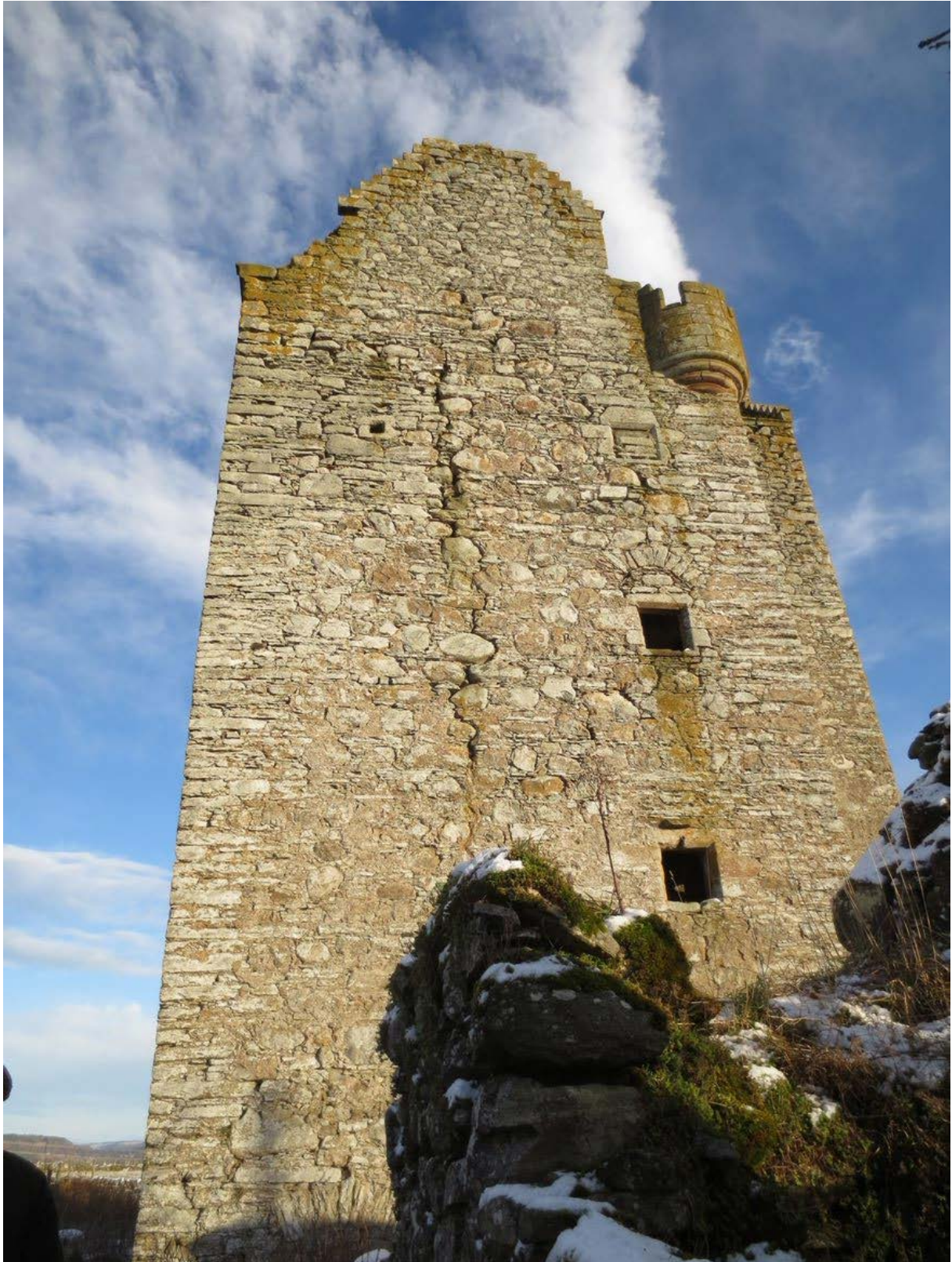
The main tower had serious cracking as well as the stair tower. The mixed quality of the rubble stone is apparent, as are some traces of the original render. Note too the window with the relieving arch, possibly used for materials access during construction.
