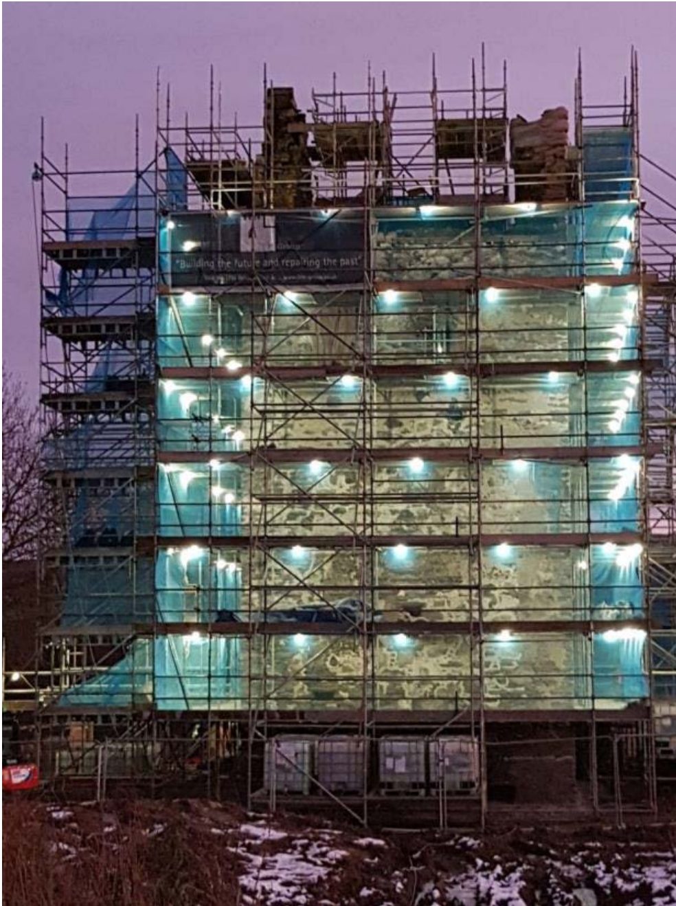
The completed scaffolding on a drear day in January 2021. The scaffold tower took more than three months to erect. It was carefully designed and placed to avoid damaging the newly discovered cobbled surface and stabilised by massive water-filled gabions.
